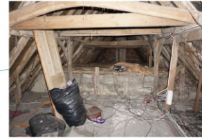
View looking through the reused aisle framing with late 17 th /18 th century rebuilt purlin roof at the far end
